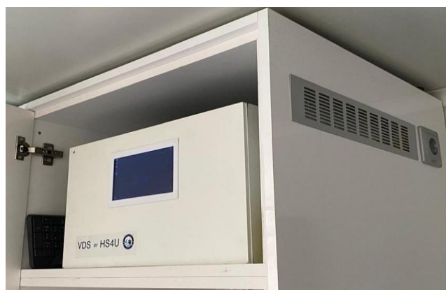
Figure 4 : VDS device installed in the Robot Cabin
