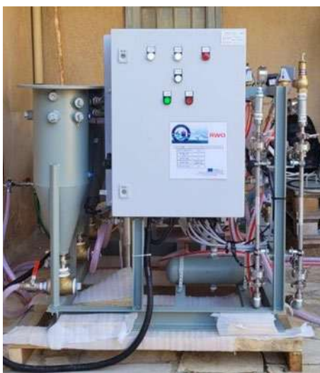
Figure 13: Wastewater epidemiological device installed in the area of demonstration
