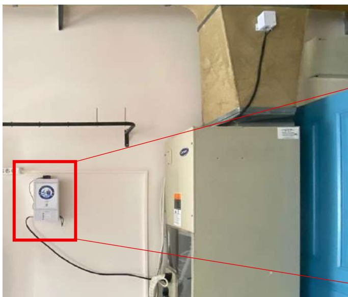
Figure 8: Wall-mounted probiotic emitter positioned in the entertainment room, connected to the HVAC system for optimal dispersion of beneficial microbes throughout the space.
